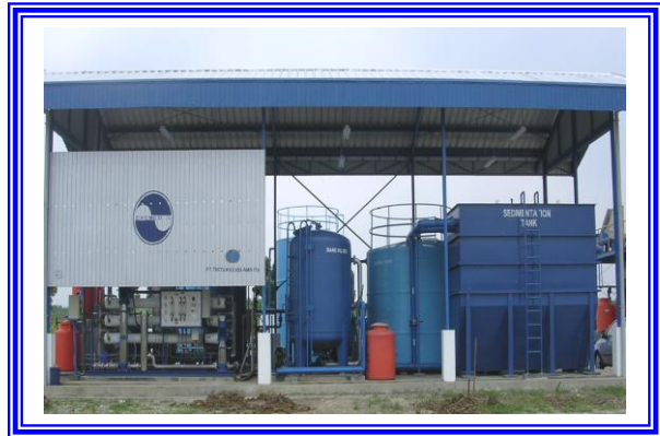
WATER RECYCLE PLANT
